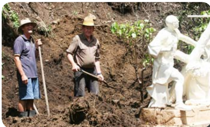
Marian Valley volunteer Robert Murphy and Br Luke doing repairs along the Stations of the Cross road after the Australia Day floods. Marian Valley received over 800mls of rain in 48 hours.
