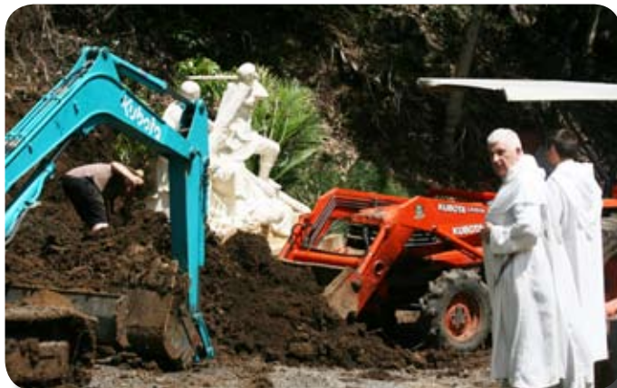
Fr Anthony and Fr Peter marvel at how the Stations of the Cross survived the landslides and watching Volunteer Tony Ryan working hard on the tractor.
